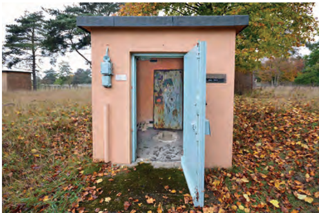
Outside the hutch, showing the replacement door (an identical replica) locking mechanism.
